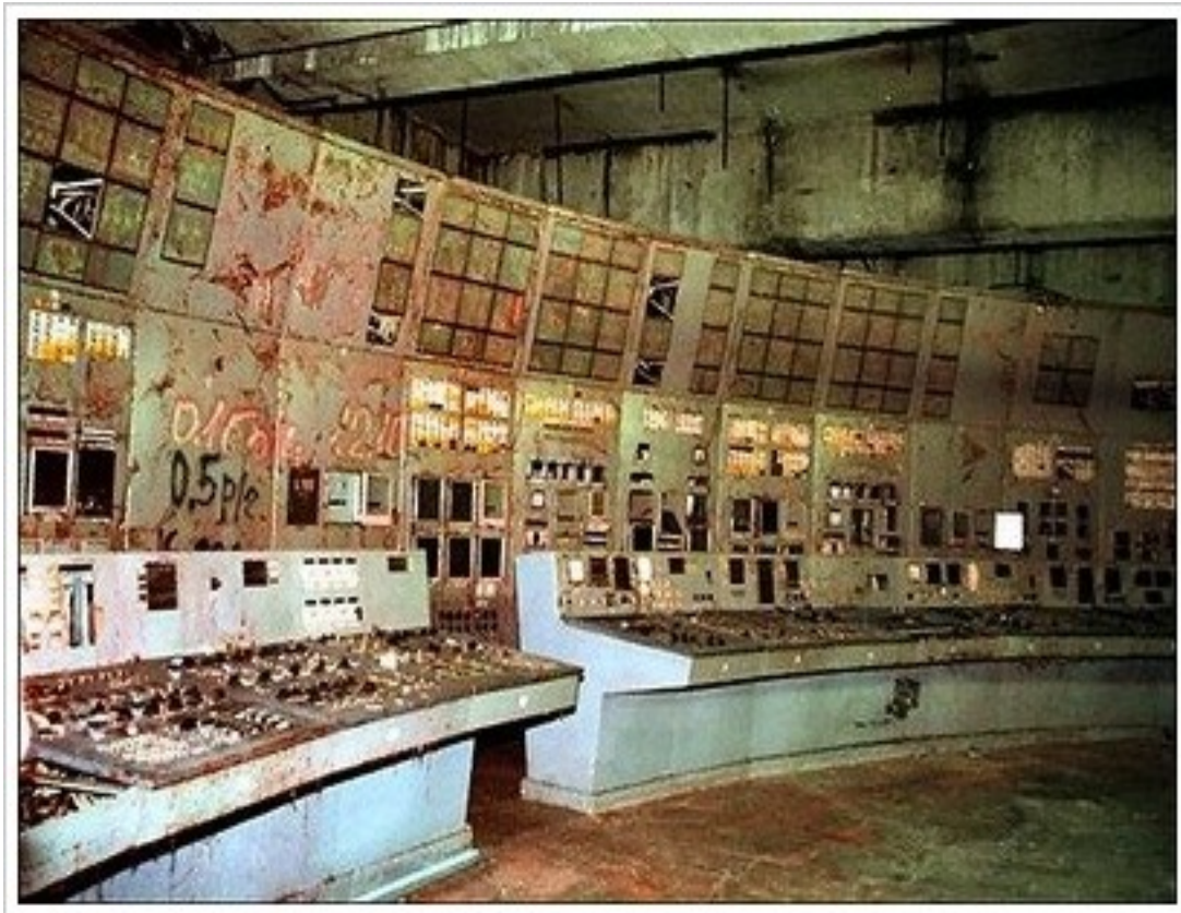
The old control room is shown inside reactor No.4 in the Chernobyl
